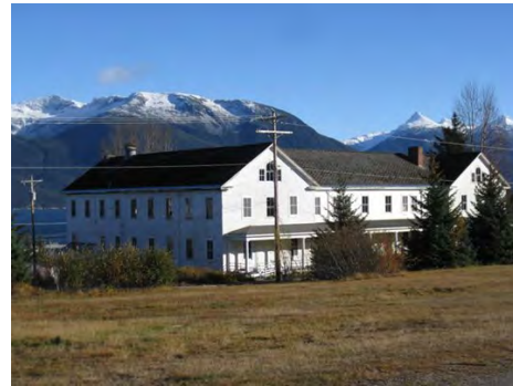
Flashing was installed around the 480 foot perimeter of the roof at the Barracks Building, Fort William H. Seward, in summer 2016.
