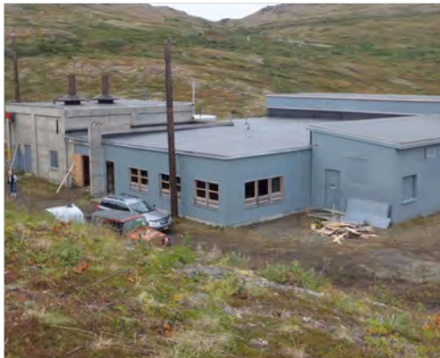
The Launch Control Building sported a new roof at the end of the 2014 work season.
