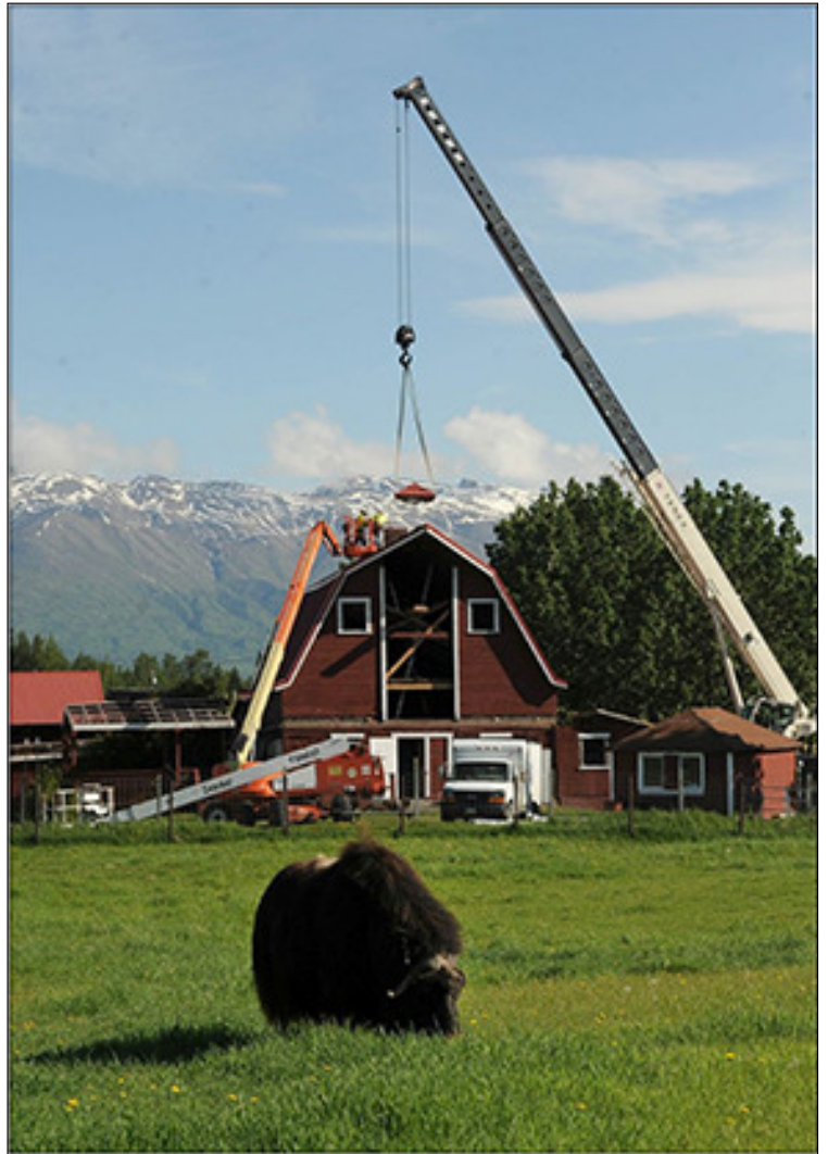
A crane lifts the roof off of the Colony barn visitors center at the Musk Ox Farm as Xavier Lechleitner helps guide it to its resting place on Thursday. (Photo by Bob Hallinen) Copyright Alaska Daily News
