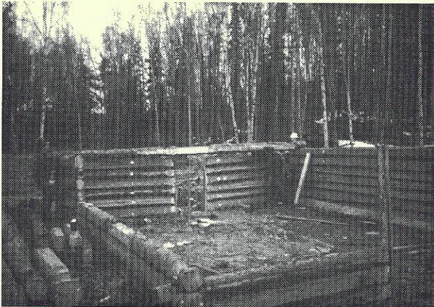
This photo, taken in mid-May at the old Sullivan Roadhouse site on Fort Greely, shows workers disassembling the main roadhouse structure.
