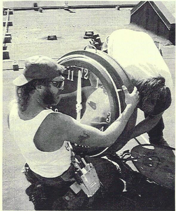
Workers recently installed the clock on the roof of Old City Hall in downtown Anchorage.
