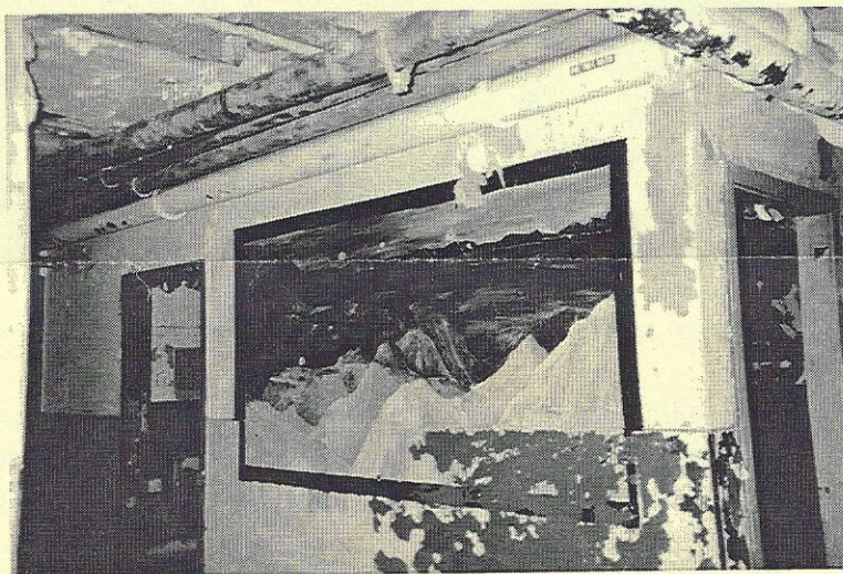
The interior of the Nike Site buildings contain a number of paintings, most of which are in a woeful state of disrepair.
