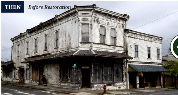
Many historic buildings face years of neglect and deterioration.
