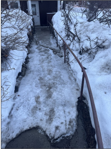
Snow and ice melting flowed down the walkway into the basement front door.
